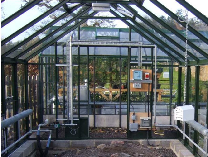
Micro Heat Installation showing controller, aspirated screen, mixing valve and pump
